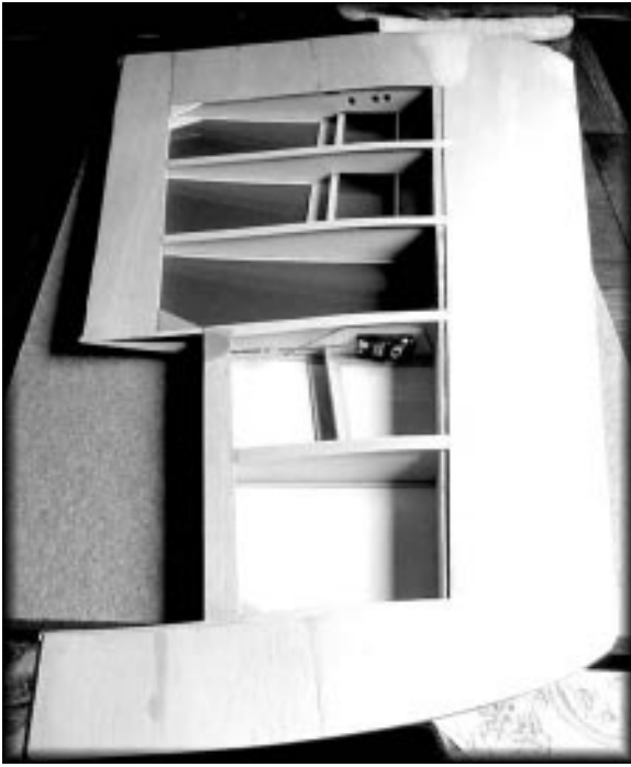
The right wing, bottom covering in place, ready for the upper surface covering to be applied. Notice the interior framing of the flap bay.
